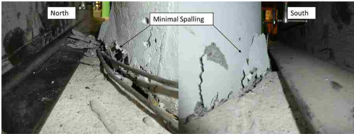
Figure 8-6. Minimal Spalling at base of column, Series 4
