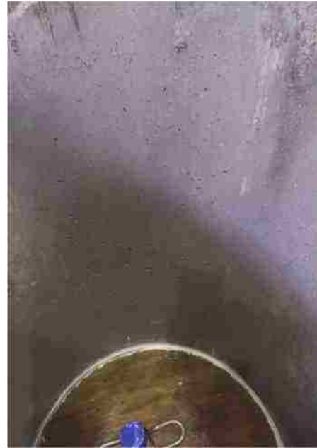
Figure 4-5. Inner surface of pipe wall without epoxy mortar
