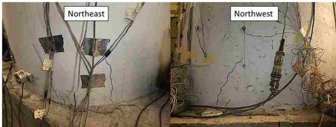
Figure 8-4. Short, fine cracks, Series 2
