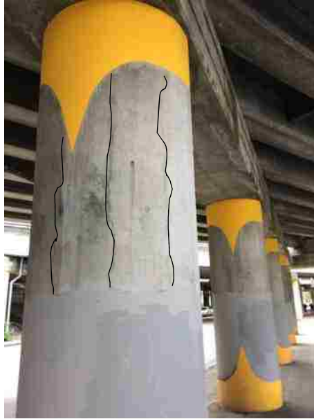
Figure 1-2. Longitudinal cracks on columns of Ravenna Bridge
