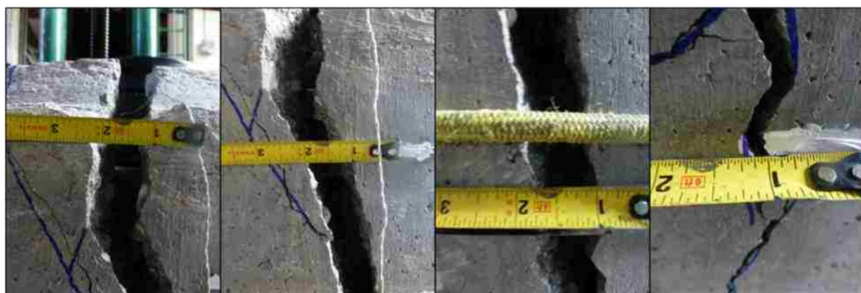
Figure 5-16. Width of large crack on west side of specimen (top to bottom)
