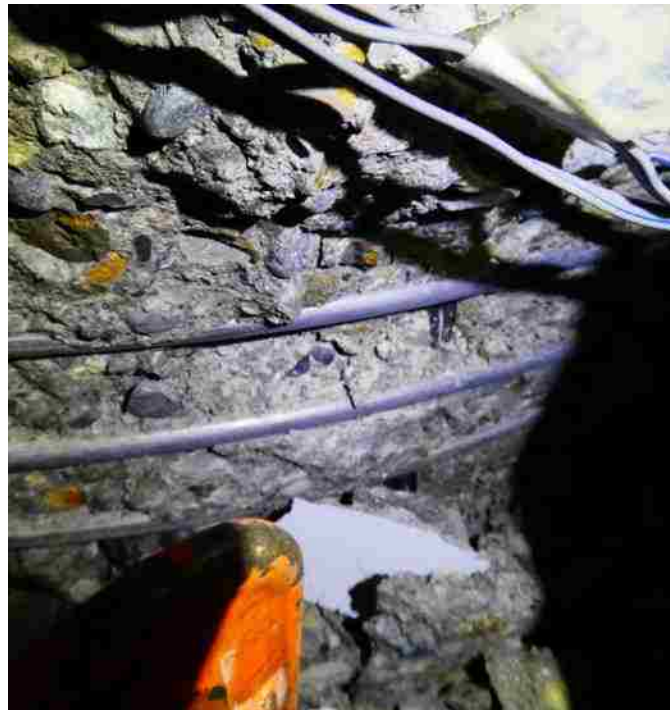
Figure 8-13. Substantial spalling and exposed spiral reinforcement, Series 8
