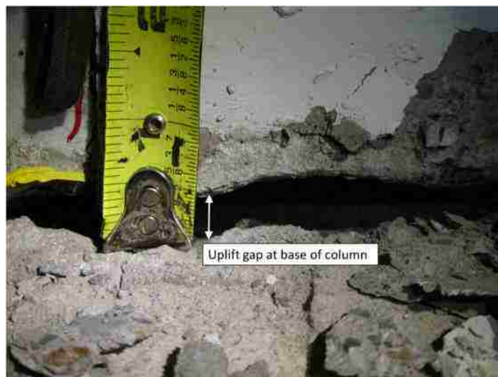
Figure 8-10. Gap from uplift at base of column measures 0.5 inches, Series 7
