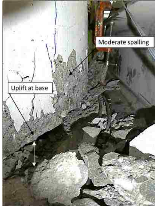
Figure 8-7. Moderate spalling and uplift on north side of column, Series 6
